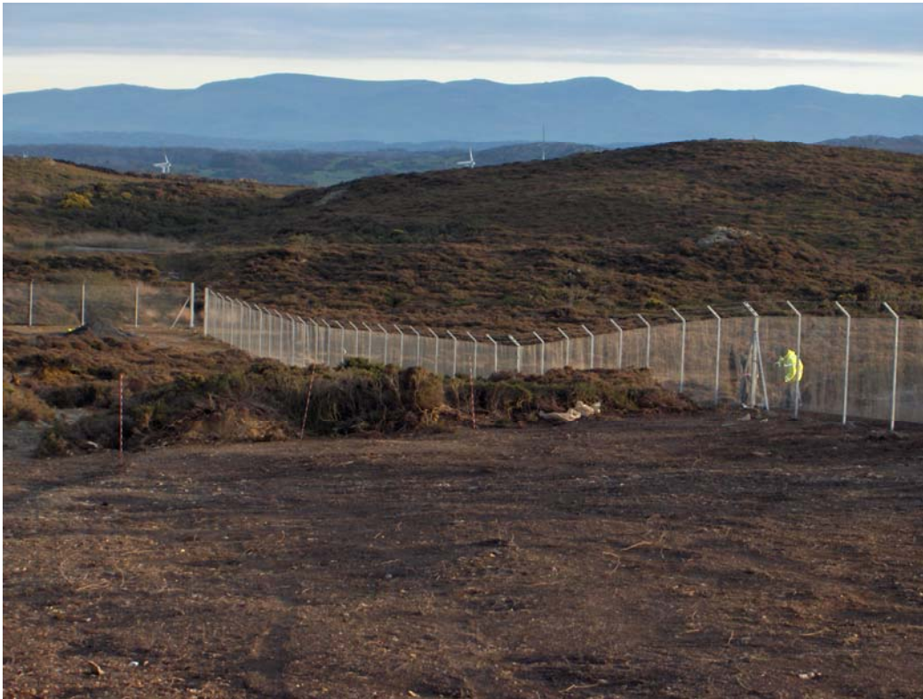
Above: Fencing around the site of the new decline at Parys Mountain in November 2007
