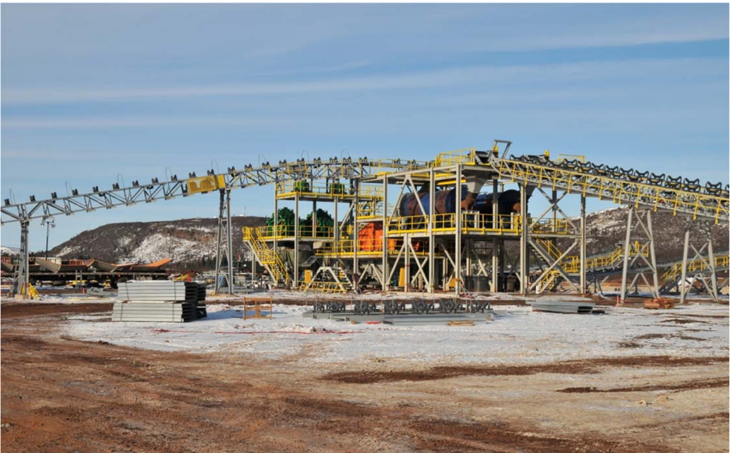
New crushing and washing plant for iron ore at the James deposit near Schefferville, Labrador
